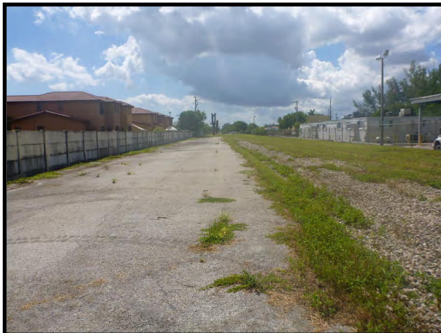
10: View of concrete patch located approximately 250 feet north of Southwest 40 th Street.
