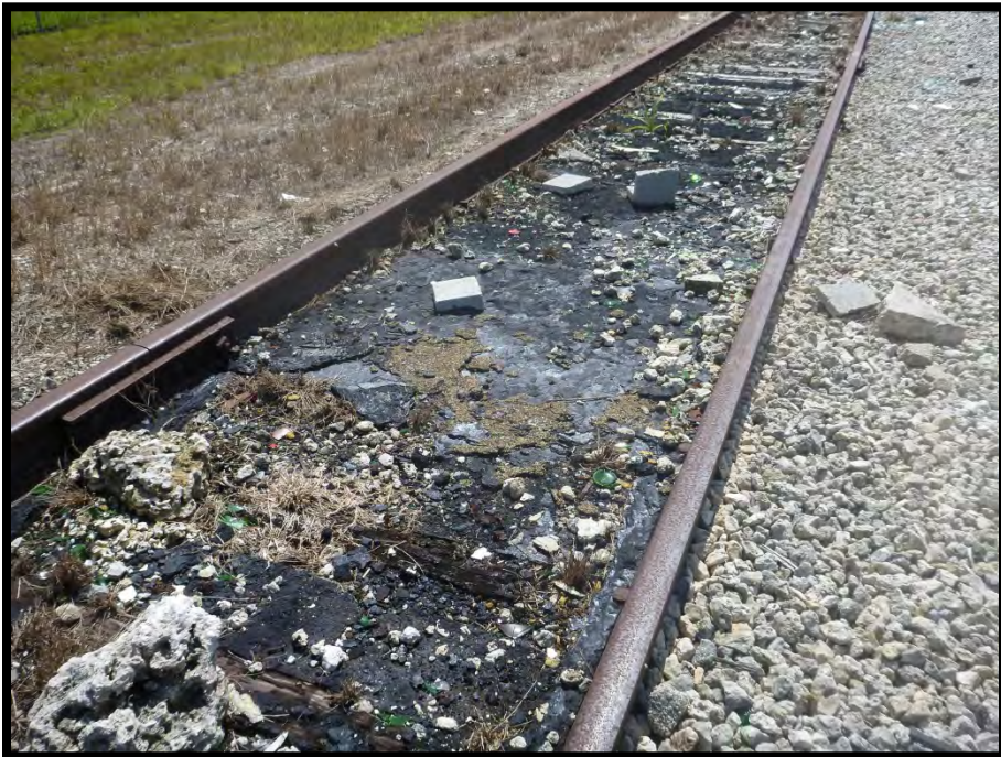
12: Stained soil located in the spur located in the vicinity of the former Dyplast.
