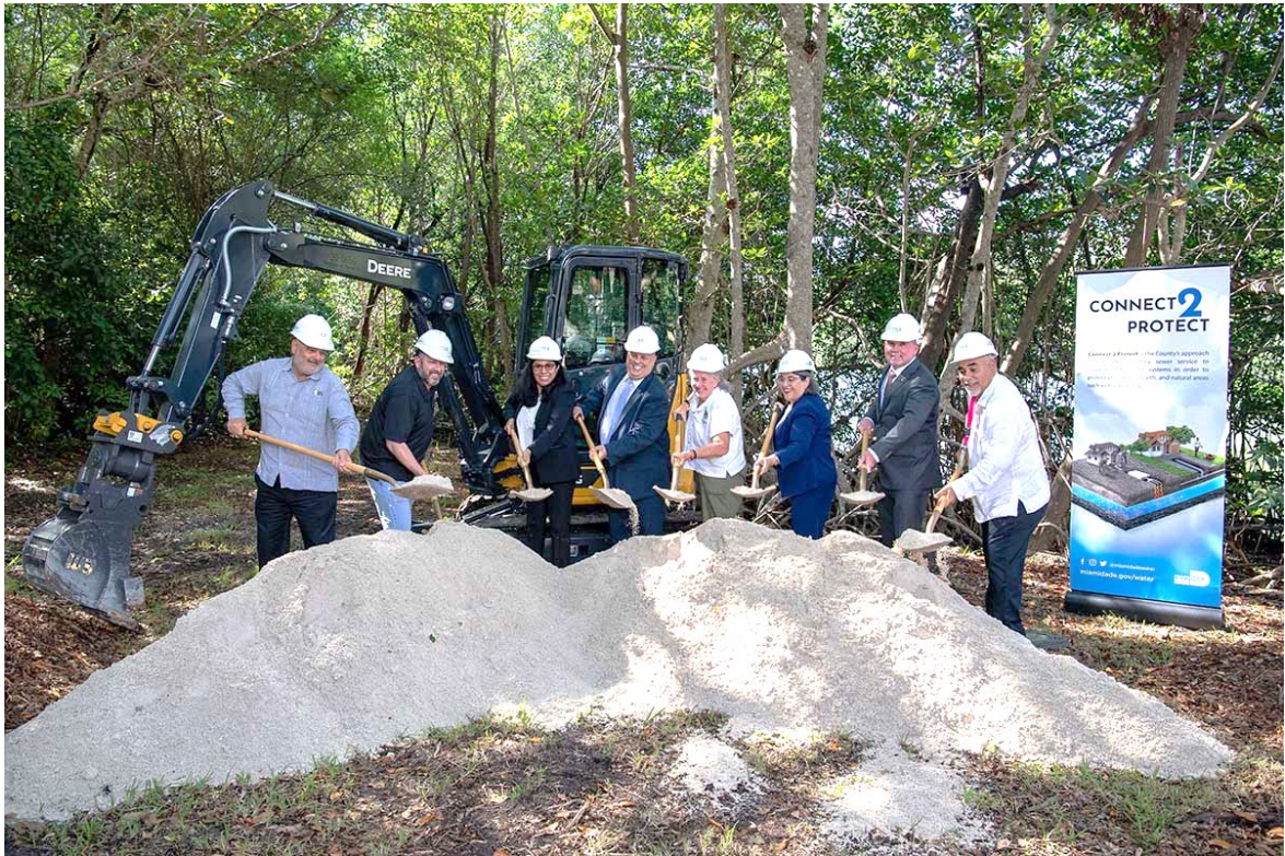
Above, the Miami-Dade Water and Sewer Department breaks ground in the Ojus Urban Area District. By expanding sanitary sewer in this area, WASD helps facilitate a more livable community through a mix of commercial and residential uses. This will not only benefit property owners and the community but also generate a positive economic impact for Miami-Dade County.
