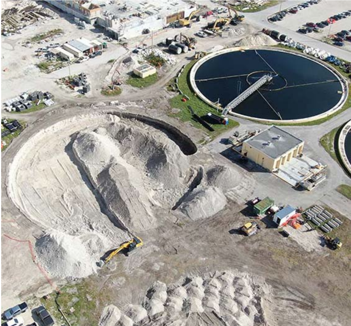
Pictured above, South District Plant Expansion Project ST-2B, Clarifiers and High-Level Disinfection, is part of the larger WASD Wastewater Treatment Plant Expansion Program, which, along with other WASD programs, is addressing aging infrastructure, redundancy, future regulations, capacity, and modernization. Additionally, Project ST-2B is creating more than 200 jobs.
