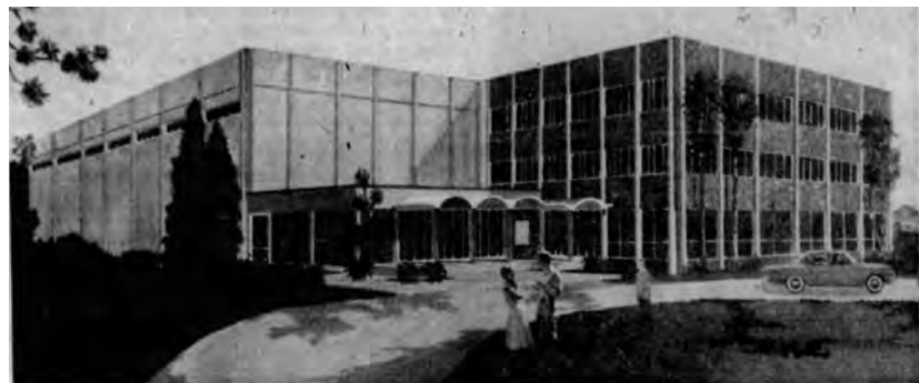
UNDER CONSTRUCTION is the new North Miami Beach City Hall and Auditorium, at 17051 NE 19th Ave. Designed by architect Ernest Wolfman, the estimated cost of the four-story building is
