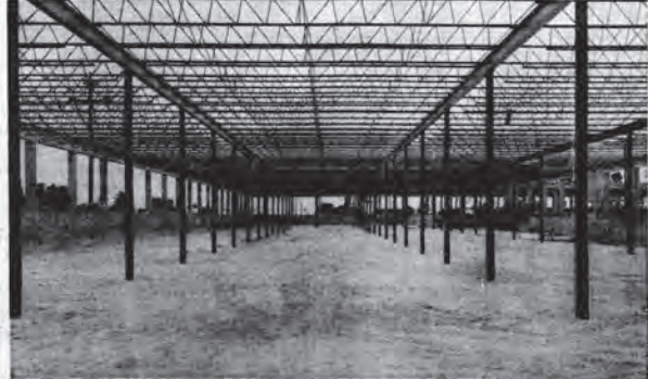
THIS 450 WING OF THE L-SHAPED BUILDING NOW BEING EQUIPPED WITH MODERN MACHINERY
