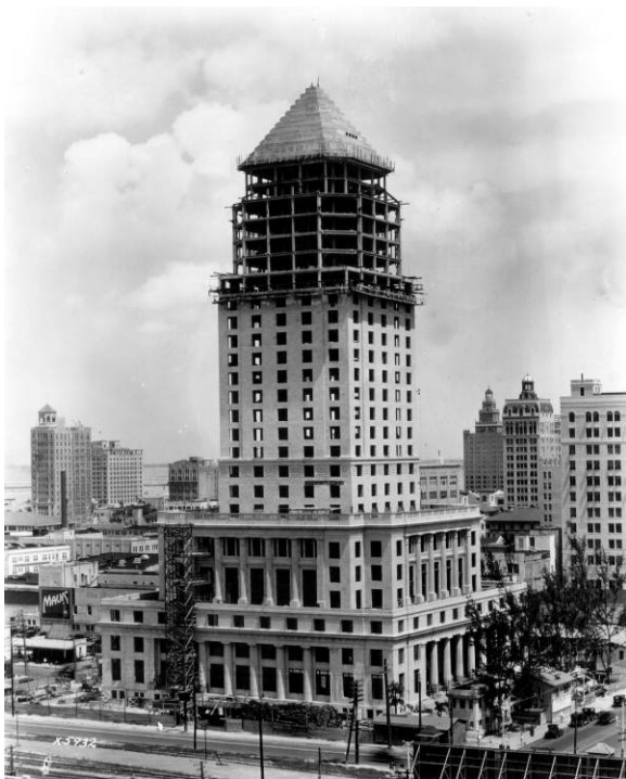
View of the Dade County Courthouse under construction in 1927. (Photo courtesy Reference Collection, Florida Memory Collection, Image No. RC10735)
