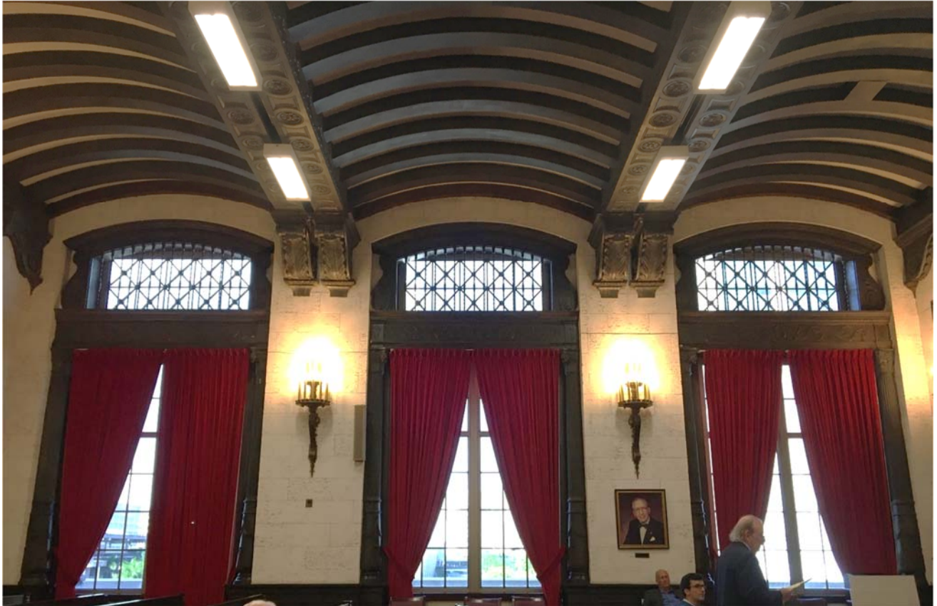
View of the domed, tripartite ceiling in Courtroom 4-2, January 2020. (Photo courtesy Office of Historic Preservation.)
