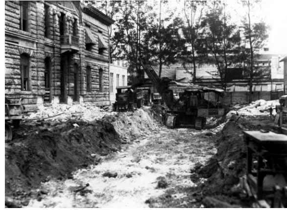
View of steam shovel being used to excavate and clear the site for the new courthouse alongside the original courthouse, visible at left, 1925. (Photo courtesy Reference Collection, Florida Memory Collection, Image No. RC19573)
