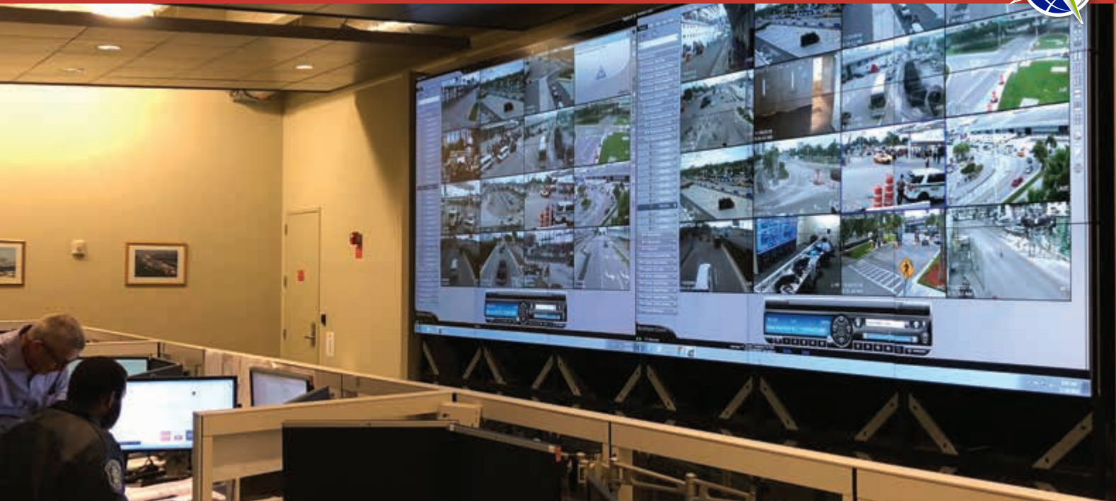
PortMiami's layered, collaborative approach to security includes a 24/7 control center offering numerous strategic surveillance camera views.
